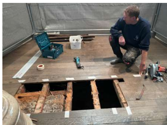
BEFORE BEGINNING THE PROJECT, WORKERS OPENED A HOLE IN THE PARQUET FLOOR TO CHECK THE FOUNDATIONS AND BEAMS. THEY FOUND LOTS OF DUST AND SPIDERWEBS – AND THE FOUNDATIONS IN GOOD CONDITION
